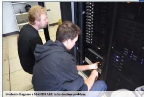
Students diagnose a MANDRAKE infrastructure problem.
